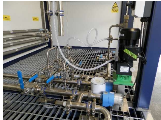
IBC Dosing Station E/2/1000 Internals
