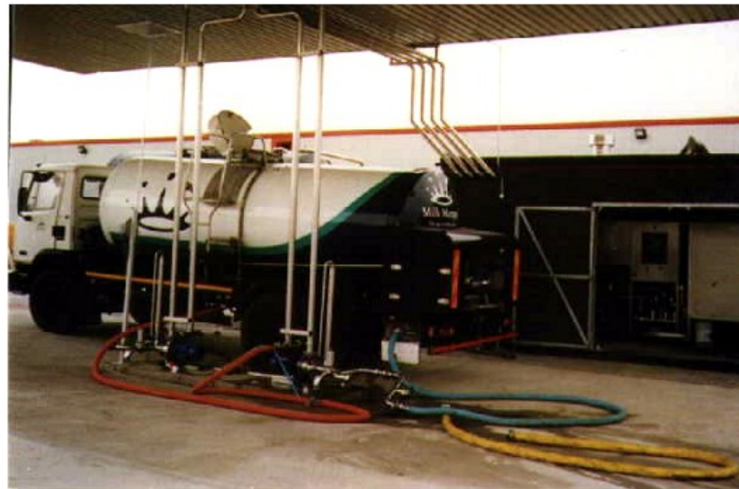
Typical Industrial Tanker Bay
